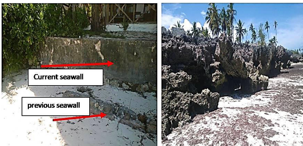
Figure 12: shoreline erosion where new seawall is built inward compared to the former at Pwanimchangani (left) and cliffs fall due to wave erosion at Matemwe (right)
